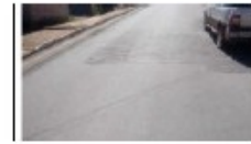
Remendo profundo 15° 38' 32" S e 58° 8' 40" W
