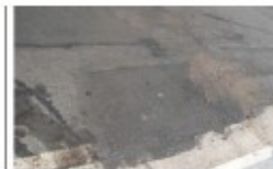
Remendo profundo 15° 35' 52" S e 56° 7' 11" W
